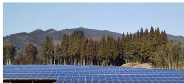
Baba Solar Power Station
